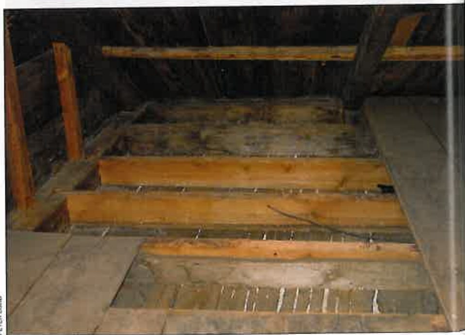
The dimensions of the bays (voids) between joists usually determine the amount of attic insulation, but it's possible to add more by raising the floor on furring.
