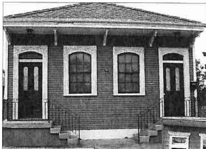
Restored original windows enhance the beauty of the House, while inappropriate replacement windows detract from the historic character and can cause future damage.
